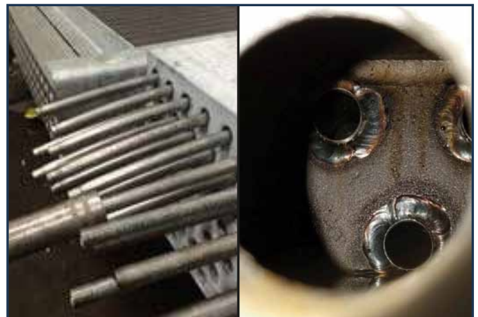
Images of full-length liners being hydraulically expanded, close up image of liner tubes trimmed to existing tube projection inside cooler header box.
