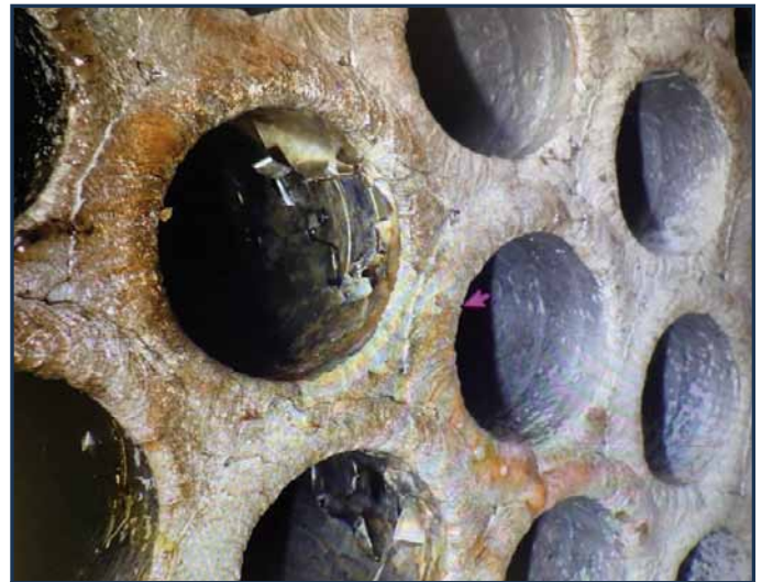
Inlet-end damage at tube-end, Curran used an alloy liner to add a corrosion barrier.
