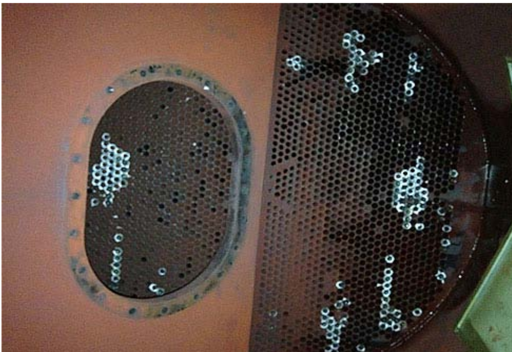
A look at desuperheater tubes sheet, about 400 tubes were found with greater than 70% surface indications. Image shows the some of the tubes marked for liner installation, most affected tubes were near extraction nozzle and impingement plate.
