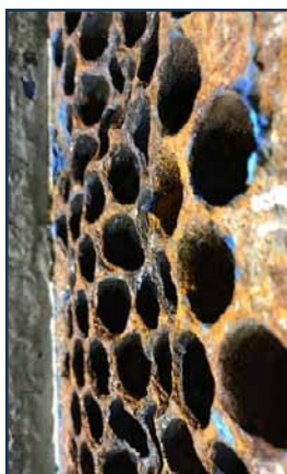
Tubesheets suffered severe corrosion, there was no cathodic protection system
