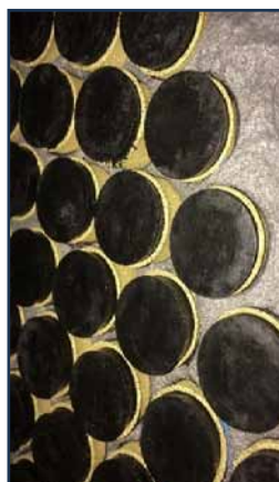
Tubesheet cleaned to "white metal," forming plugs set to gauge coating thickness.
