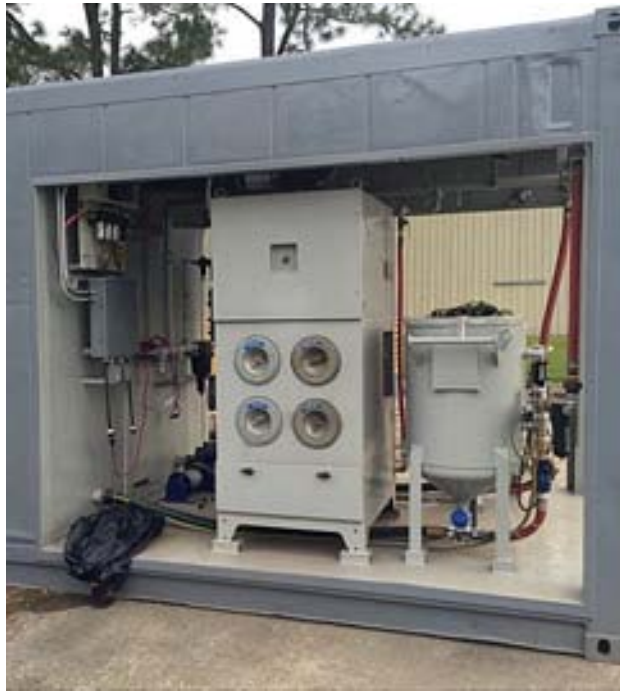
Utility end of tube cleaning module with integrated dust vacuum, sand pots.
