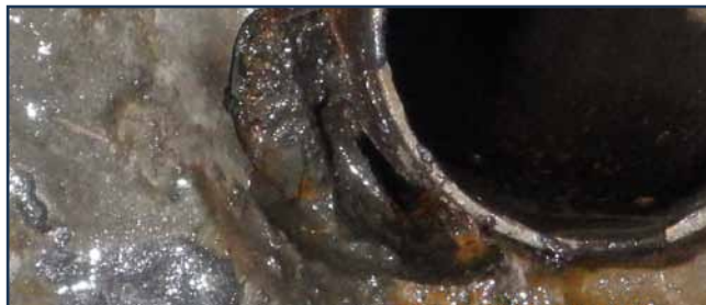
Hole at the Tube to Tubesheet Interface
