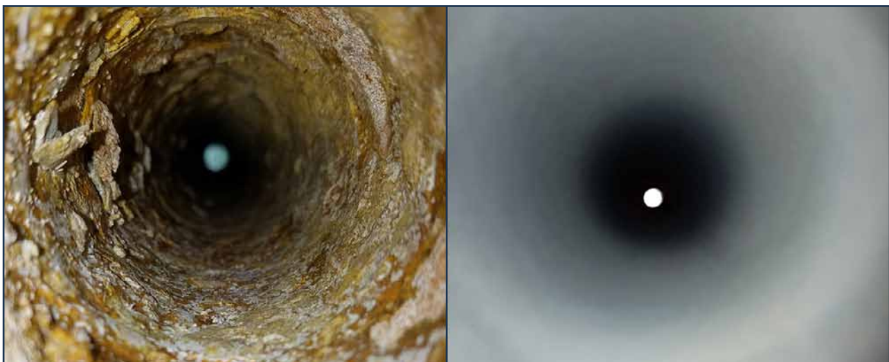
Image of fouled tube ID (L) in sulfur service: risk of under deposit corrosion and impact heat transfer; grit blasted tube (R) facilitates accurate NDE, and returns heat transfer duty. Dry grit does not react with sulfur waste debris, and is highly containable.
