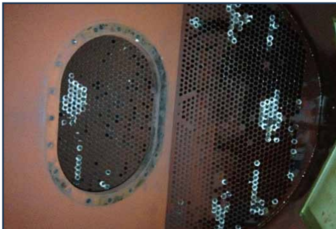
Desuperheater exchanger, image shows the tubesheet where about 400 tubes with greater than 70% surface indications and required repair liners were found. The image also shows tubes marked for repair.
